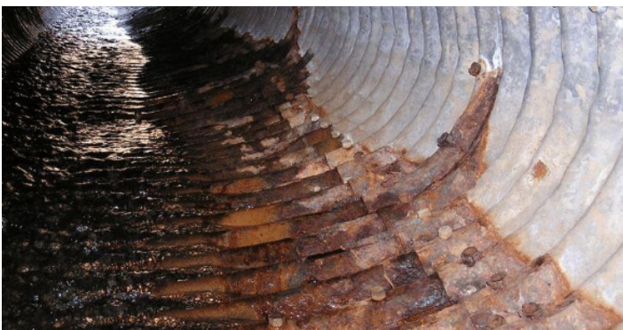
Failing metal pipe located on Glenwood Creston
