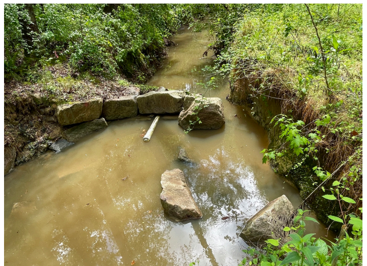
Damaged in-stream structure at Millbrook Exchange Park
