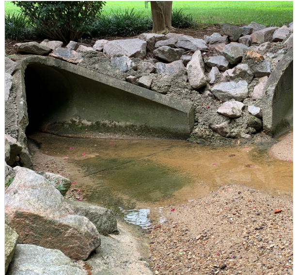
Stormwater pipes at Western North Ridge
